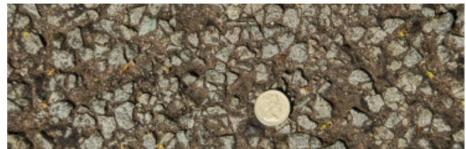
Worn road surface with aggregate raised above bitumen matrix £1 coin for scale
